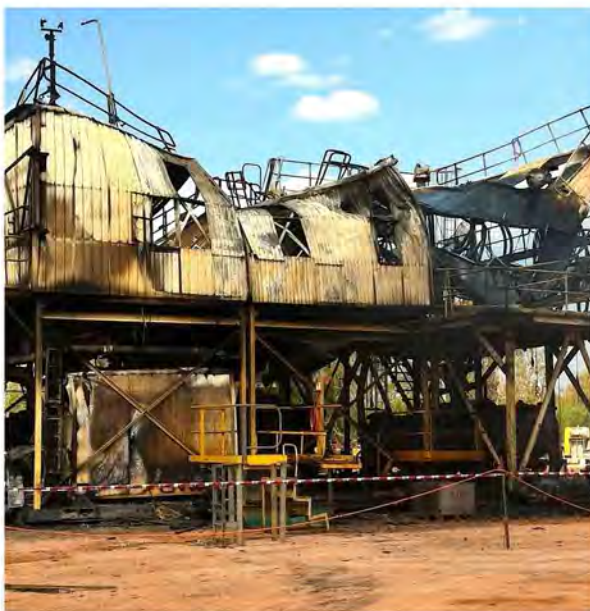
Tragic fire - the concentrator plant destroyed in 2011
